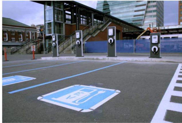
Figure 7: PEV Parking Stall with Recommended Symbol on Pavement vi
