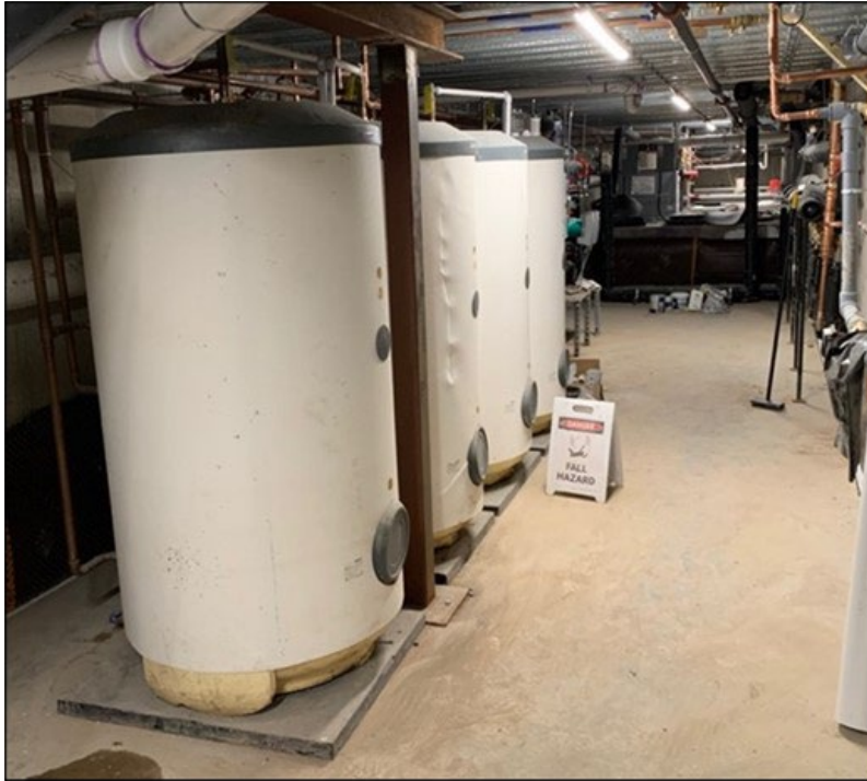
Figure 6. Photo of the DHW Tanks in Basement
