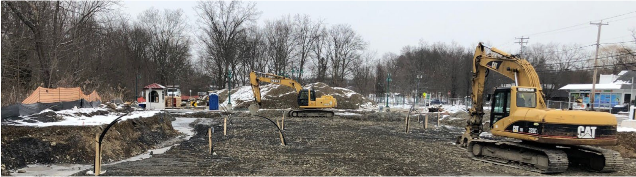
Figure 4. Photo of the Vertical Bores Installed Before Building Construction (the bores used only 15% of the building footprint)
