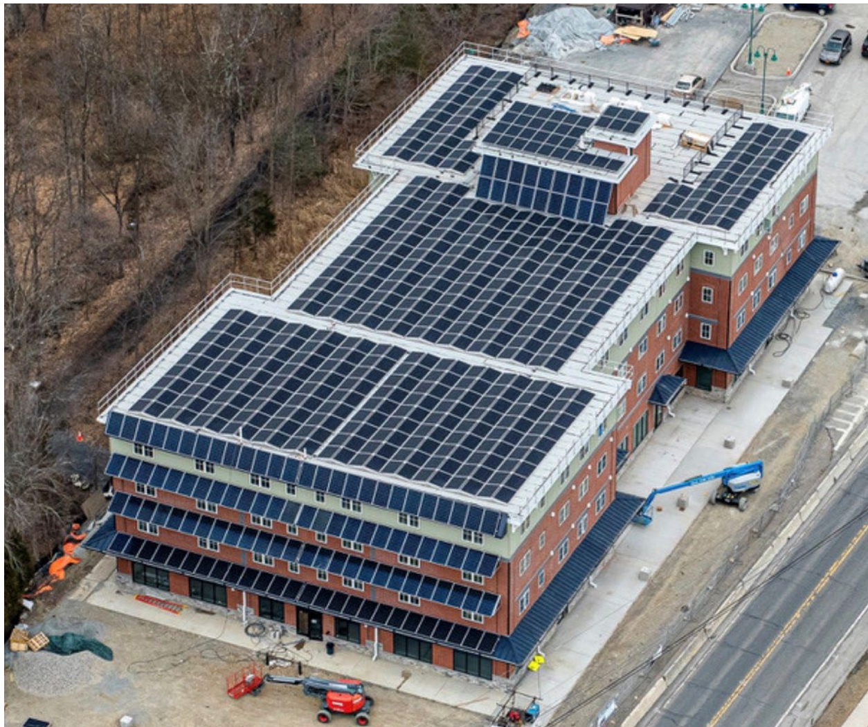
Figure 3. Photos of 248 kW Solar Array on the Building Roof
