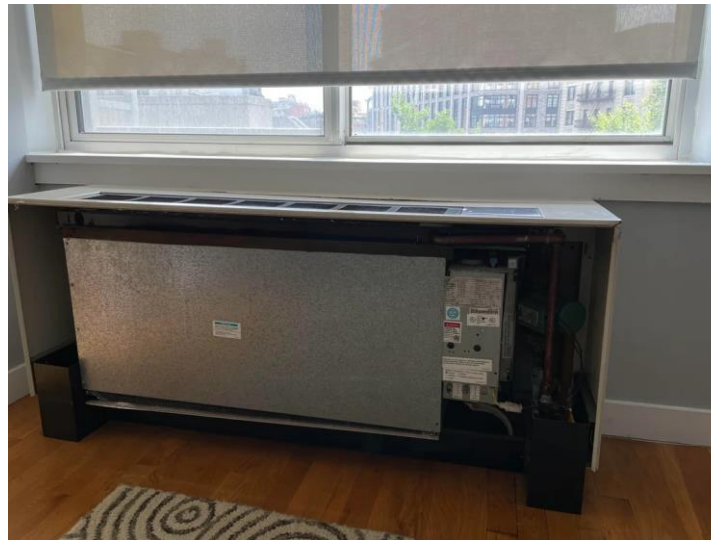
2. Hydronic Heat PTACs
