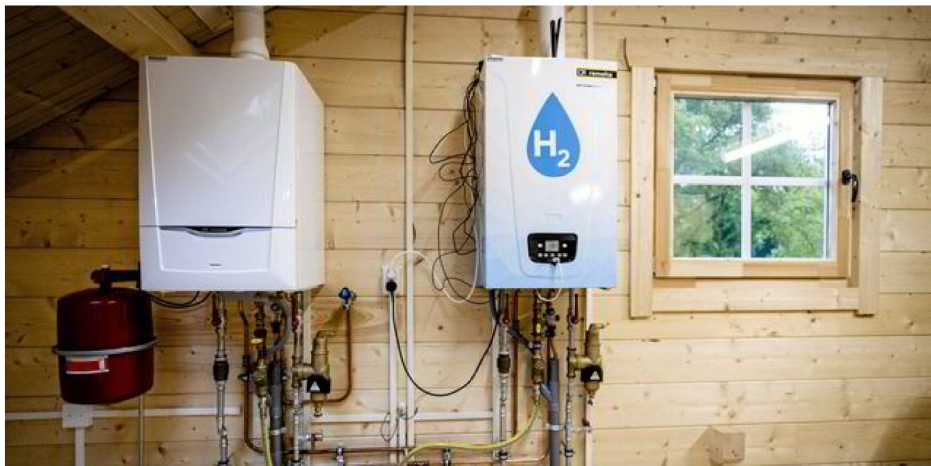
An old central heating boiler (L) and a hydrogen boiler inside the Hydrogen Experience Centre in Apeldoorn, Netherlands, the hydrogen house of certification body Kiwa and Dutch gas, heat and power distributor Alliander Photo: AFP/Getty
