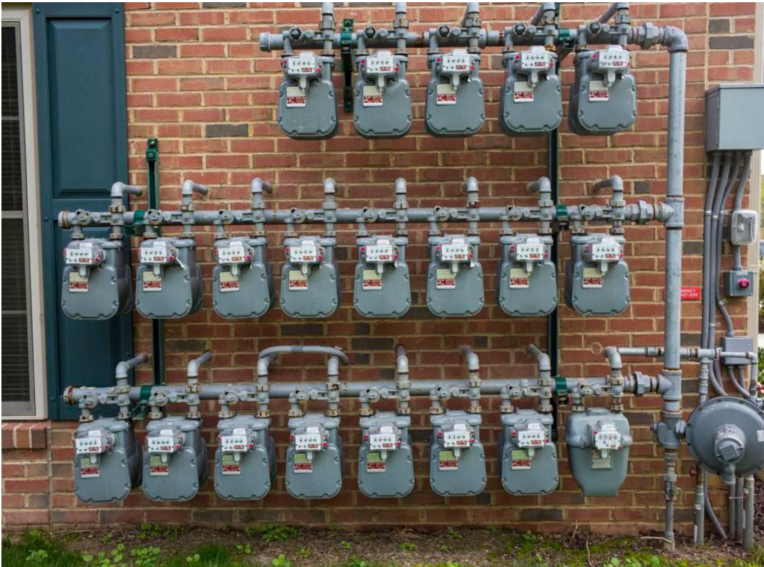
Natural gas meters are fixed to the outside of residential townhouses and apartments at a building ... [+] GETTY IMAGES
