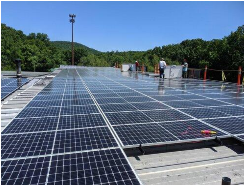
Figure 2. Ecogy’s community solar 301 kW DC system rooftop of the Village of Croton-on-Hudson on the Department of Public Works building.
