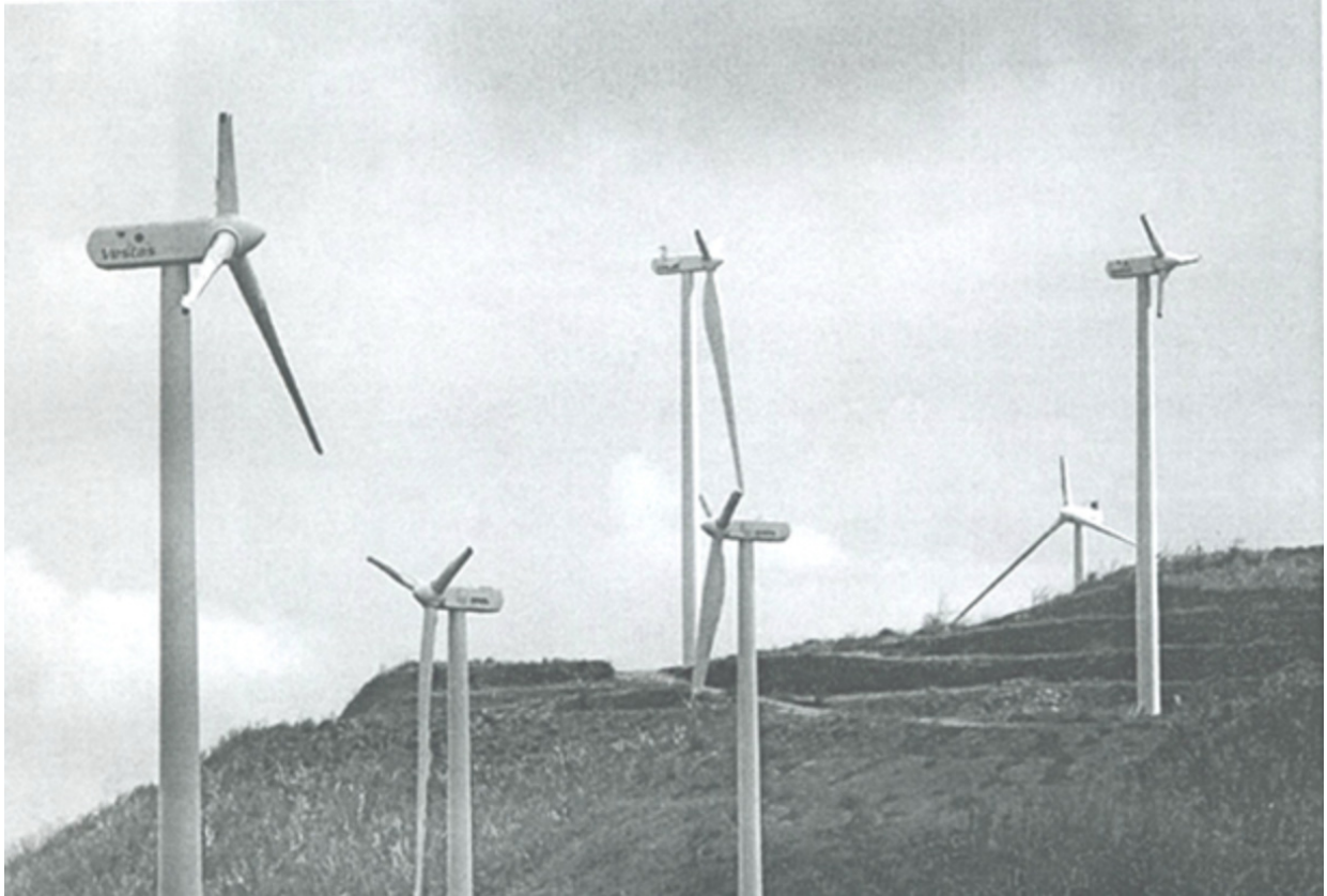
FIGURE A-4 Impact of Hurricane Maria on Wind Turbines in Puerto Rico
