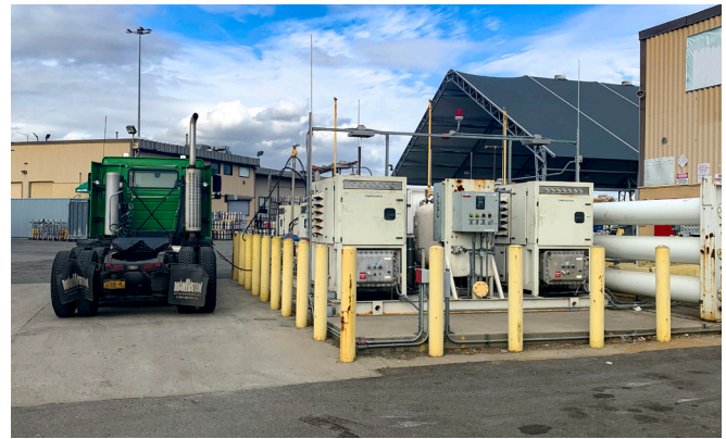
CNG tanks and pumps at Manhattan Beer Distributors
