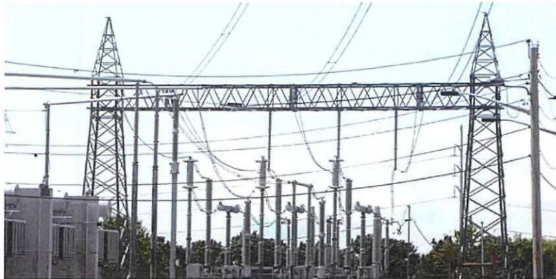
Power transmission lines run from the northern terminal of the Cross-Sound Cable, seen here in 2003, which has been out of commission since July. Credit: Bloomberg News / Steven E. Frischling
