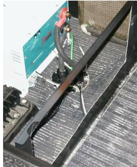
Figure 16: Hole cut in passenger's side partition wall for the Intellitec distribution panel.
