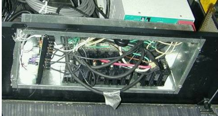
Figure 45: Completed Intellitec wiring (cover was removed for picture)
