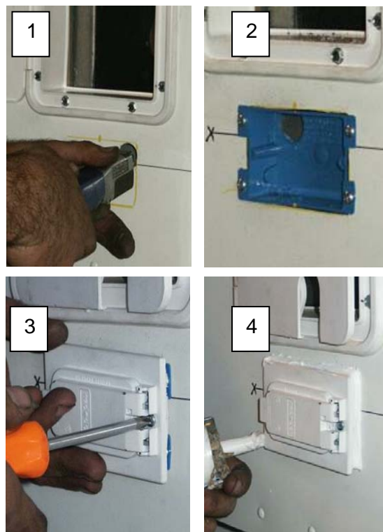
Figure 34: Internet connection receptacle installation
