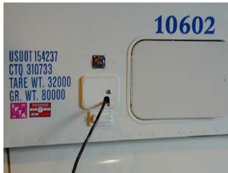
Figure 1. Phone/ Cable/ Internet receptacles, and Shorepower line access
