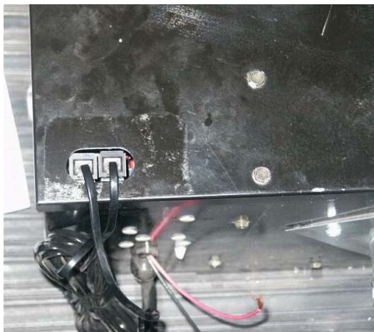
Figure 9: HVAC remote control panel control wire connector
