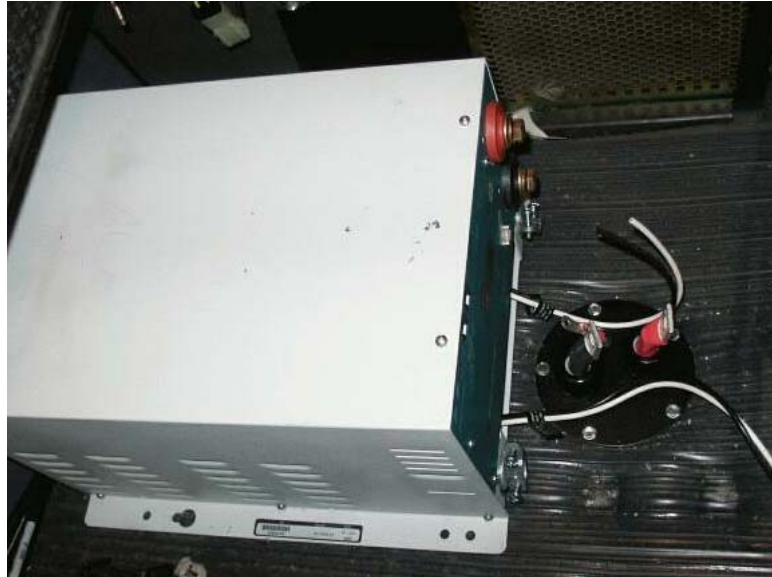
Figure 12: DelcoRemy mounting plate attached to floor with battery cables routed through, but not attached to inverter
