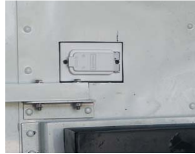
Figure 11. Exterior 120-volt receptacle located at rear of cab
