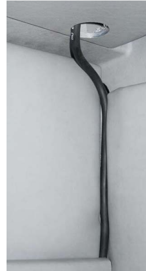
Figure 26: Semi-concealed electrical outlet wiring run
