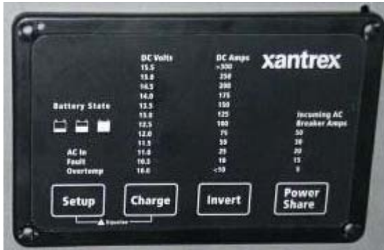
Figure 15: Xantrex inverter Freedom Link remote control panel
