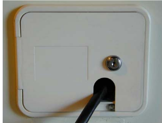
Figure 31: Close up of the locking RV electrical hatch used for the main power connection
