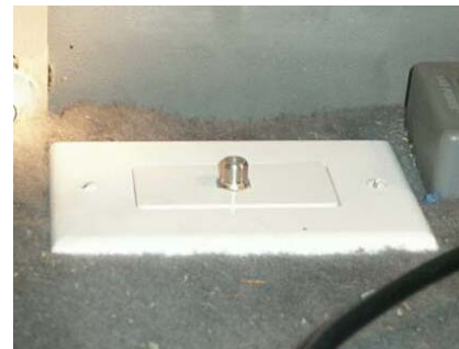
Figure 37: Cable TV wall plate mounted on floor of TV area
