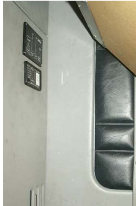
Figure 20: Front view of inverter and Intellitec remote panel mountings
