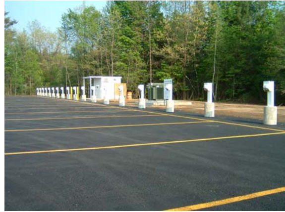
Figure 6. Newly Installed Shorepower Facility at the Wilton Travel Plaza
