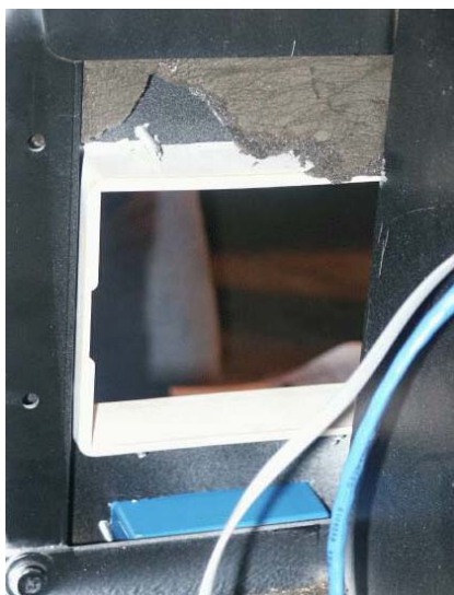
Figure 35: Interior shot of Internet electrical box installation
