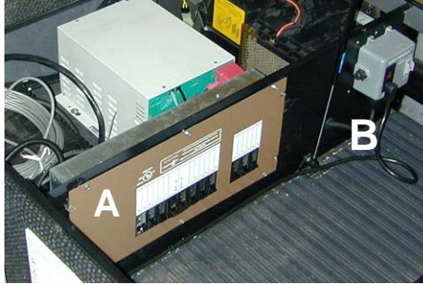
Figure 13. Intellitec breaker panel (A) and HVAC outlet (B) located under the bunk
