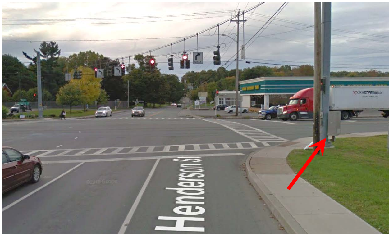
Figure 4. Example Intersection Showing Auxiliary Cabinet (Henderson Street and Commercial Drive)
