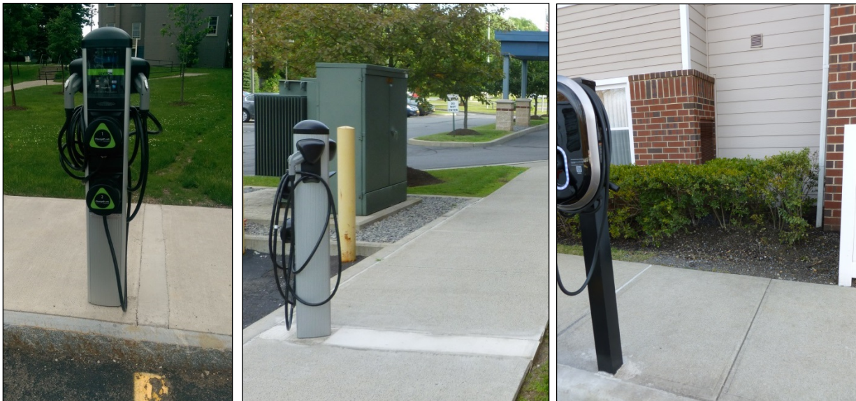
Figure 17: Concrete walkway examples of cut/repair (left and center) and tunneling under (right)
