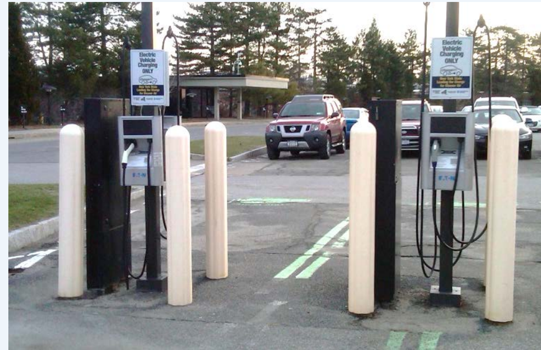
Level 2 Charger at IBM in Ossining
