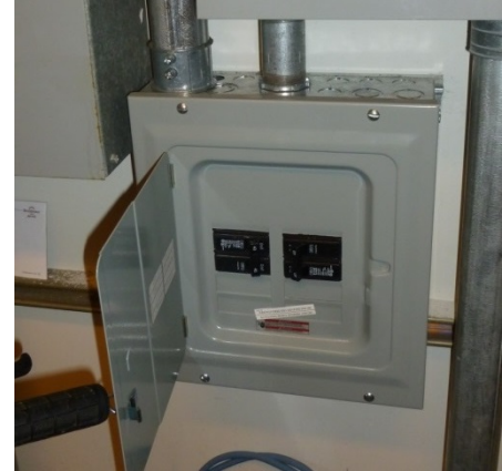
Figure 12: Added subpanel for charging station circuits
