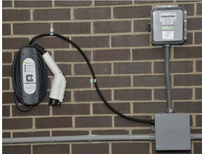
Figure 4: AC Level 1 charging station
