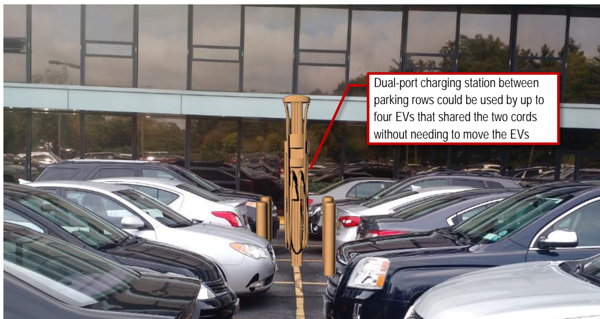
Figure 6. Potential EV charging location at Treeline Properties on Ring Road in Garden City beside building 100 and between parking rows
