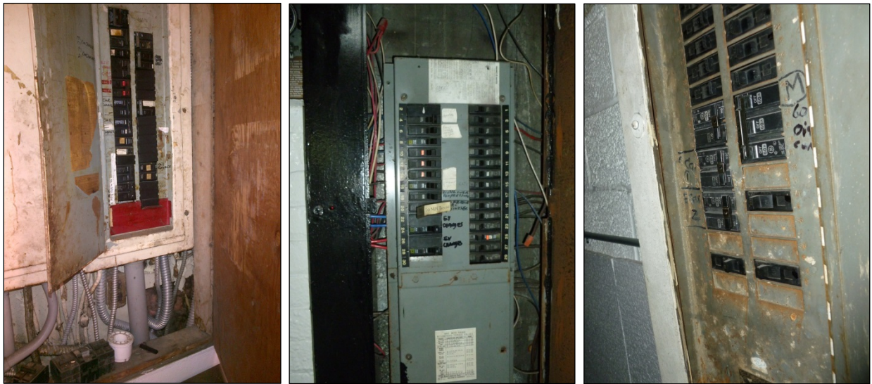
Figure 10: Older electrical panels may require upgrades to bring up to modern codes
