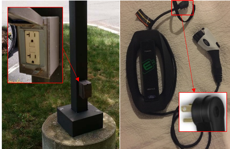
Figure 5. Outlets, such as these on light poles (left) can be offered for EV charging using an EV driver's portable connector (right) if they are on an individual circuit
