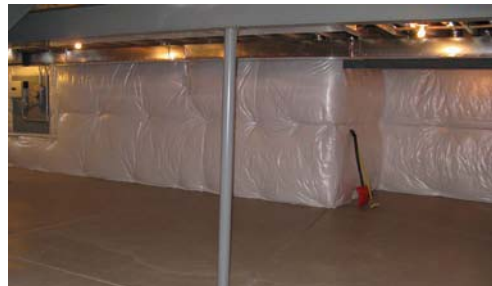
R-26 Fiberglass batts with a perforated facing mounted on basement foundation walls
