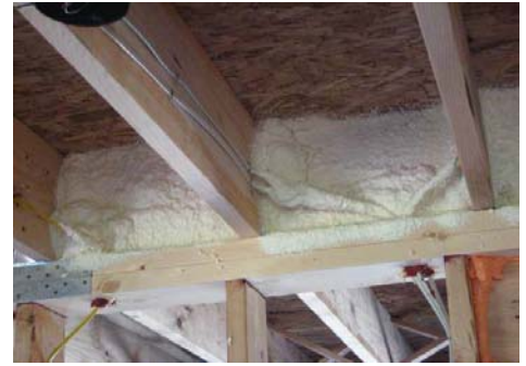
Isolating the ceiling system of garage from adjacent family room with spray foam
