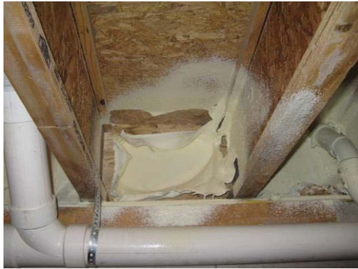
Spray foam in rim joists that shrank instead of expanding
