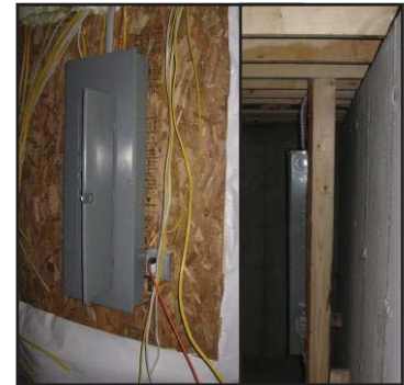
Electrical panel built away from wall to allow for insulation behind it
