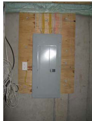
Electrical panel built away from wall to allow for continuous insulation
