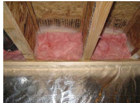
Full length blanket insulation with spray foam and fiberglass batted rim joist in the basement.
