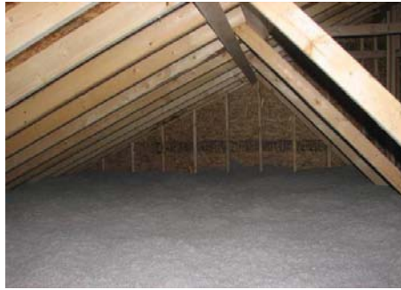
R-50 (16") blown cellulose in attic
