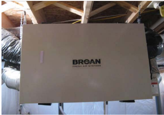
HRV unit in the basement, which distributes fresh air throughout the house through the central duct system
