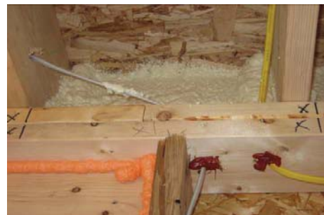
Air sealing using spray foam in band joist (which will also be insulated with a fiberglass batt), and caulk and foam at penetrations and framing joints.
