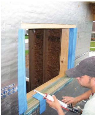
Sealant was applied before setting windows. Note the 2” x 2” board around rough opening perimeter.
