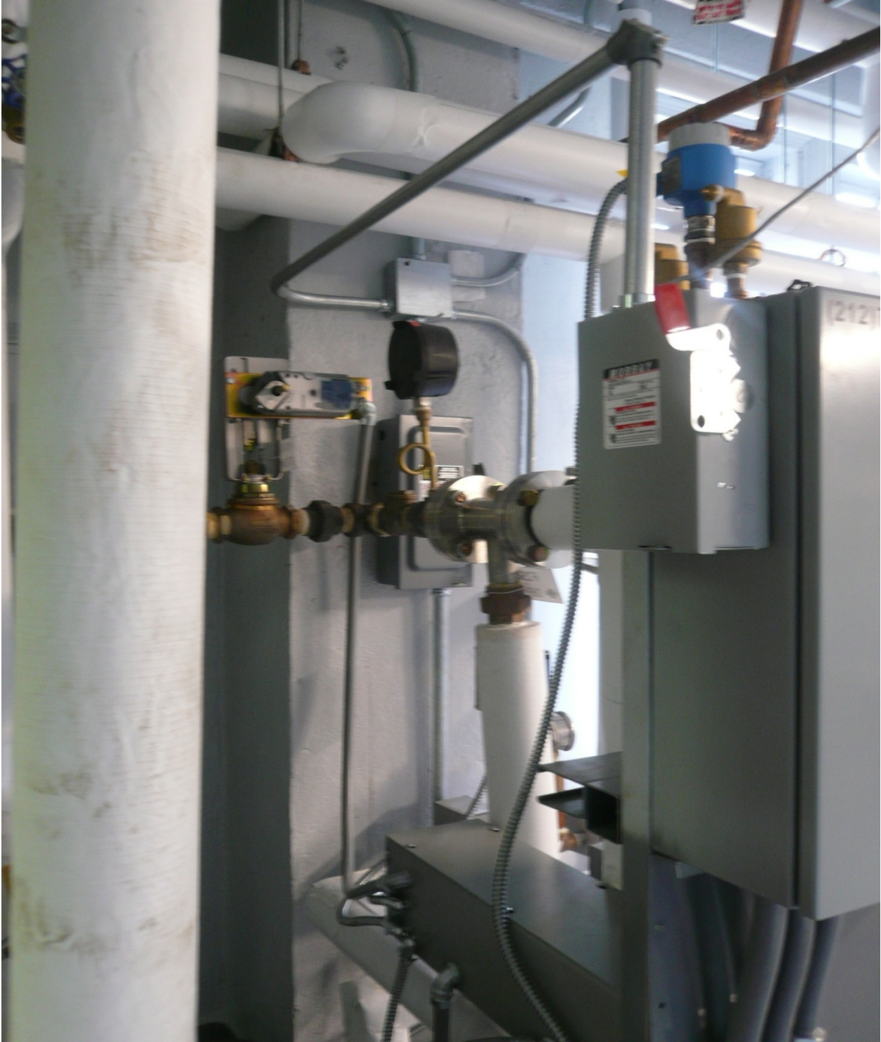
Figure 43. The Control and Data Recording Package of the New DHW Unit
