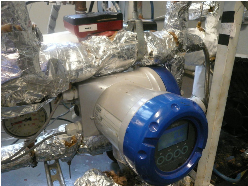
Figure 34. Overall View of the Flow Meter
