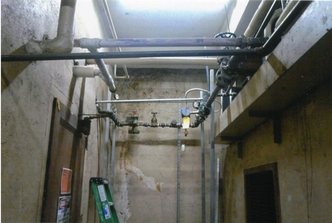
Figure 11. Con Edison Steam Supply to Test Facility
