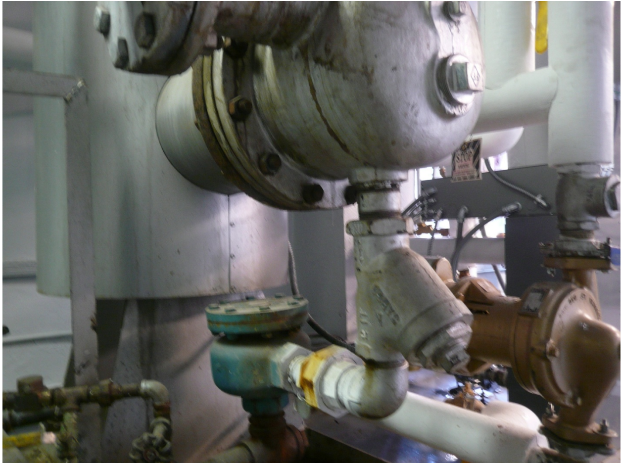
Figure 38. Steam Condensate Drain of the Existing DHW unit
