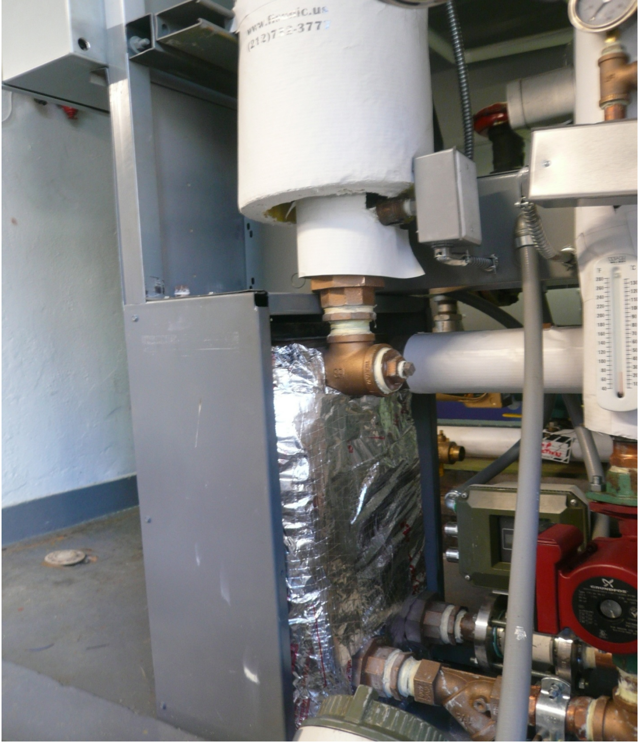
Figure 42. Brazen Plate Heat Exchanger of the New Unit
