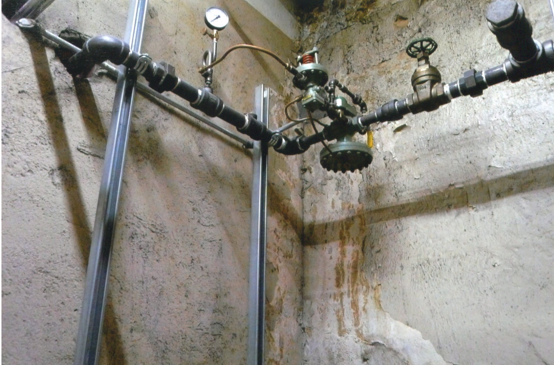
Figure 12. Steam Pressure Reducing Valve
