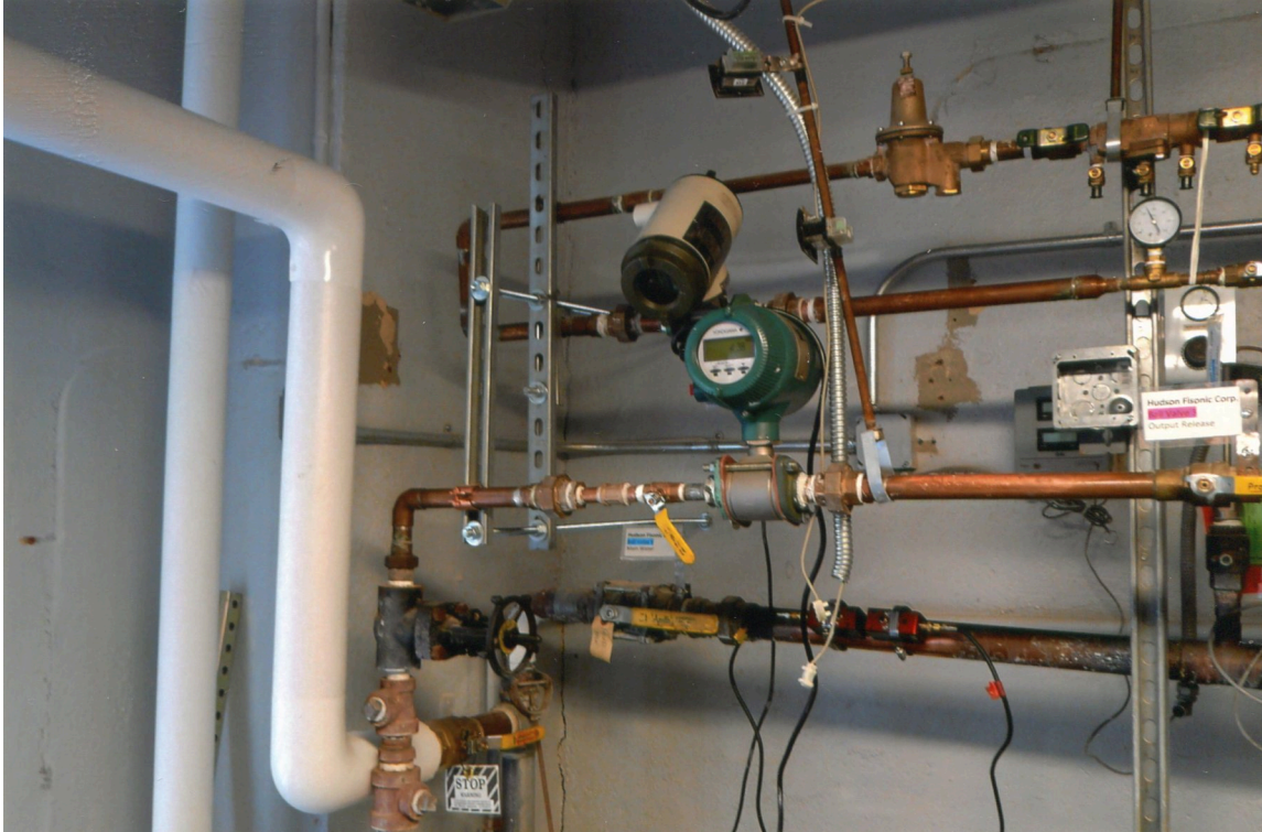
Figure 14. Cold and Hot Water Flow Meters
