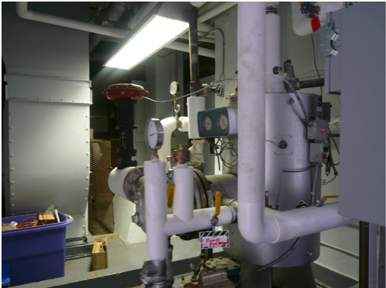
Figure 35. Front View of Existing Patterson Kelly 400 Domestic Hot Water Unit
