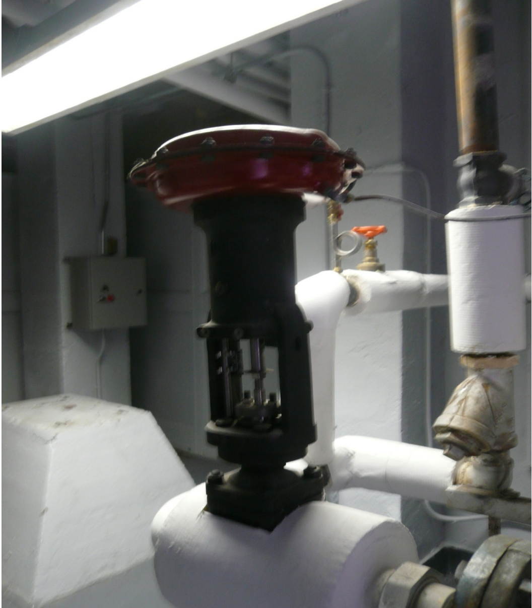
Figure 37. Steam Control Valve of the Existing DHW unit
