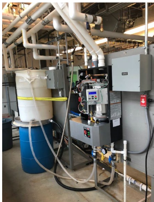
Figure 7. Residential Boiler Installed at Syracuse Center of Excellence in Environmental and Energy Systems (SyracuseCoE) with Dummy Heating Load
