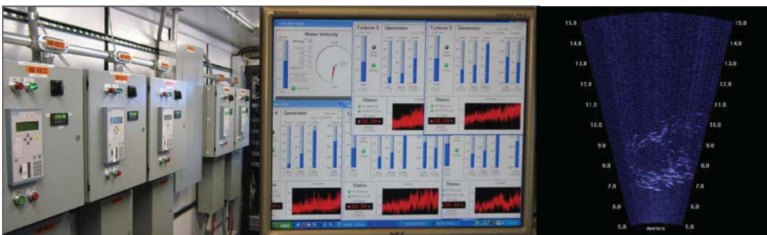
Fig. 7 – RITE Project Control Room equipped with Switchgear, Turbine Data Acquisition System and Environmental Monitoring Equipment
