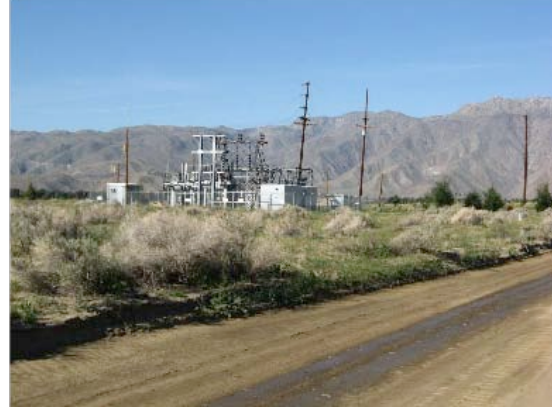
Figure A2: SDG&E's Borrego Springs Substation
