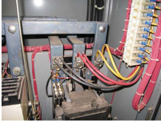
Figure 27. Close Up View of Wiring to the USES Devices
