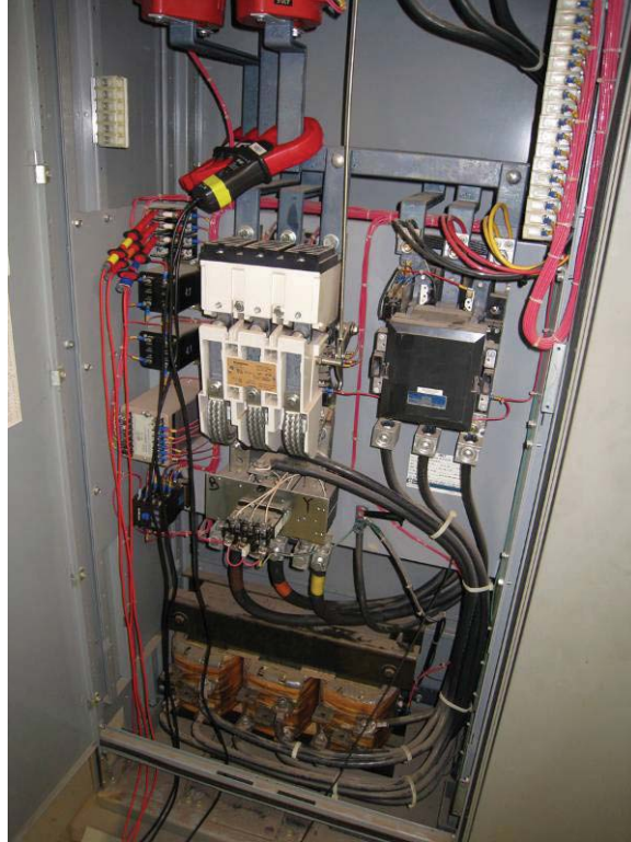
Figure 30. Location of the Test Probes (Note that the Cables were Routed through the Lower Kick-Panel that was Removed During Testing)
