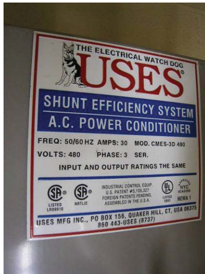
Figure 21. USES A.C. Power Conditioner Label
