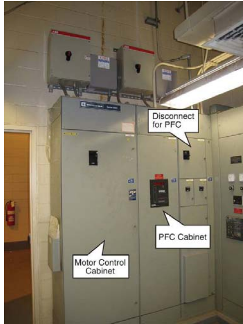
Figure 25. Exterior of 186 kW Motor Control Cabinet (The Two USES Devices can be seen above the Motor Control Cabinet)
