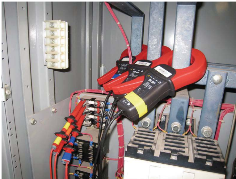
Figure 31. Detail of Probe Location on Bus Bar. Terminal Block used for Voltage Monitor Probes was Verified to be Wired to the Main Bus Bar by Visual Inspection and by using an Ohmmeter.
