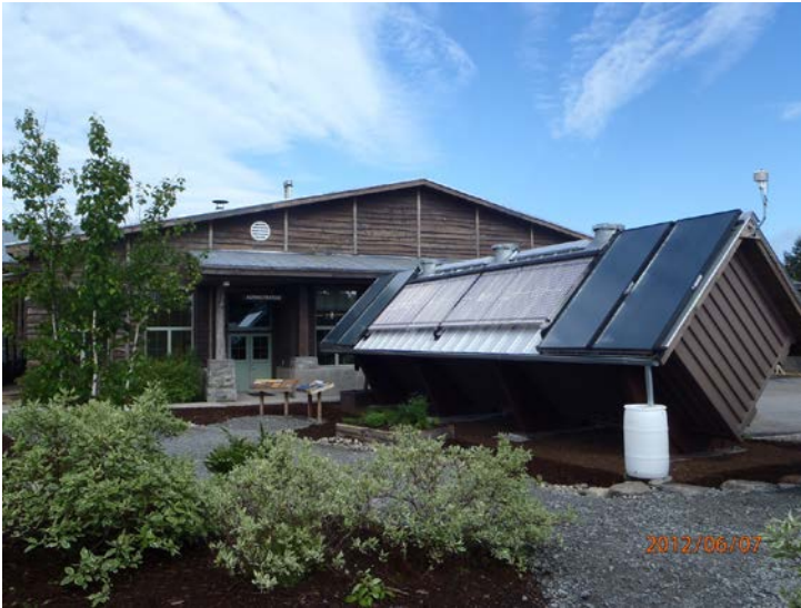
Figure S-4. Solar-thermal plate collectors and evacuated tubes are mounted on the roof of the pellet storage container at the Wild Center.
