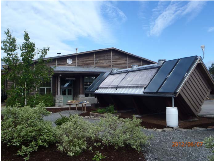
Figure S-4. Solar-thermal plate collectors and evacuated tubes are mounted on the roof of the pellet storage container at the Wild Center.
