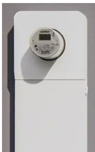
Smart electrical distribution panel
