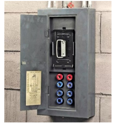
Fuse box style panel
