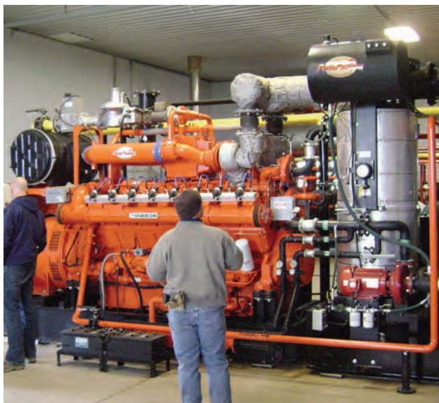
Biogas Generator – NYSERDA photo
