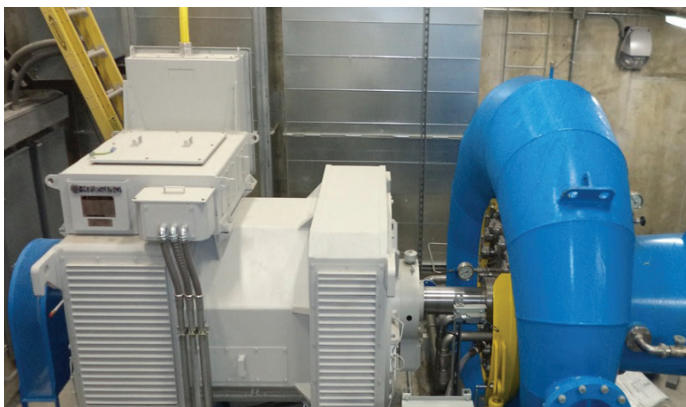
Rio Hydroelectric Bypass Flow Unit, Sullivan County, NY
