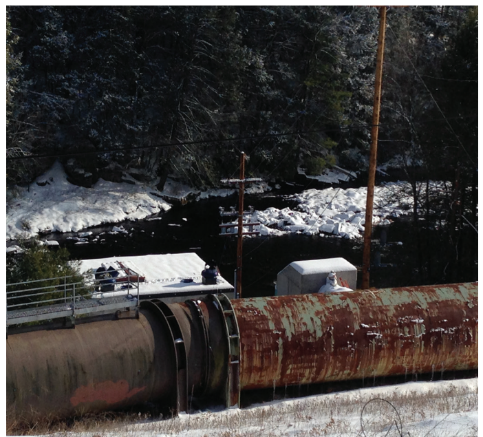
Rio Hydroelectric Bypass Flow Unit, Sullivan County, NY
