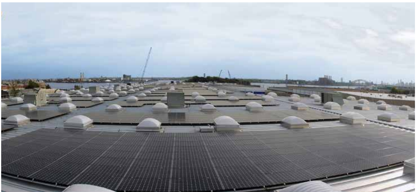
Jetco Cash and Carry, Bronx County, NY Photo Courtesy of Solar Design Associates
