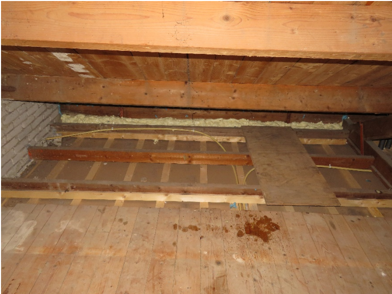
Figure A36: Attic in renovated building showing evidence of air sealing, but the insulation is all exterior, above the roof-line
