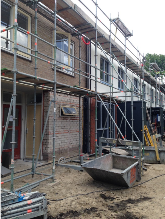
Figure A15. A closer look at the existing façade and scaffolding for renovation
