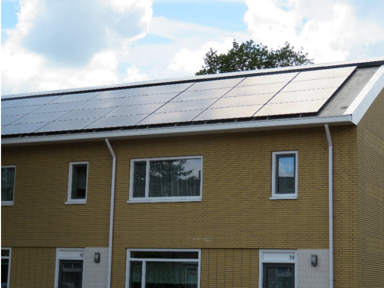
Figure A40. Solar modules on roof
