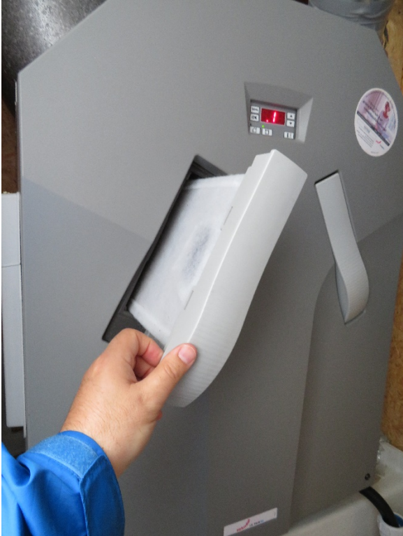
Figure A8. Filter in heat recovery ventilator
