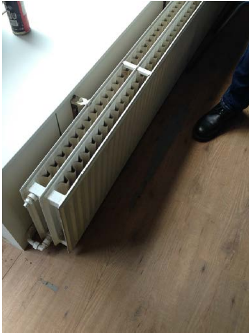
Figure 3. Radiator left inside the building
