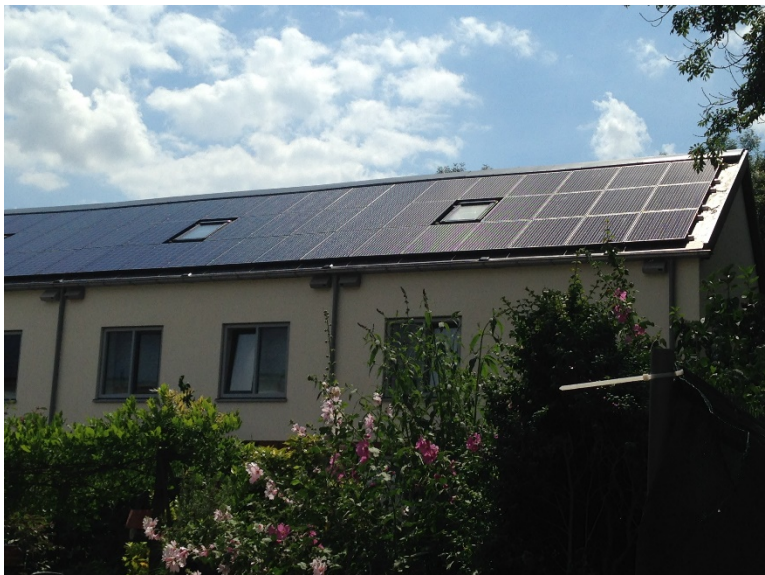
Figure 4. Solar photovoltaic installation
