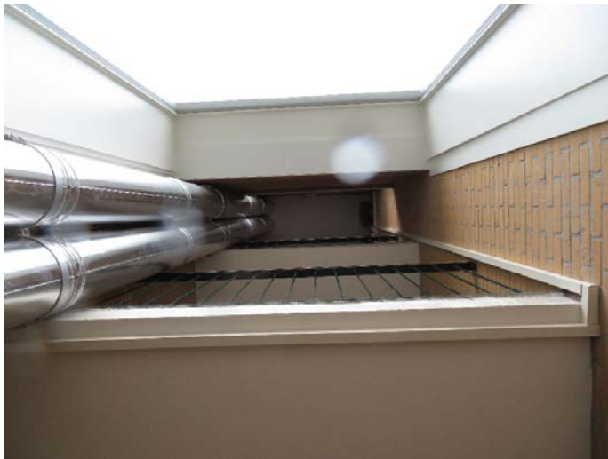
Figure A29. Ventilation ductwork in renovated building
