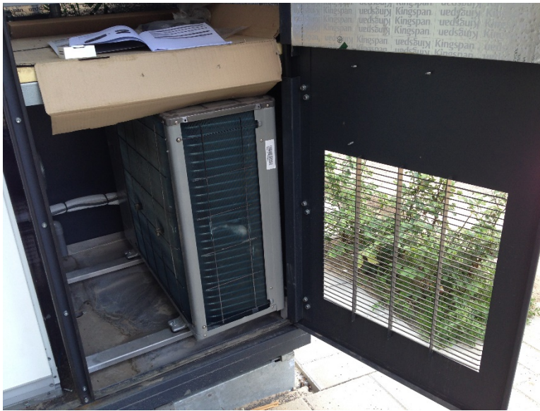
Figure 5. The outdoor fan and heat exchanger
