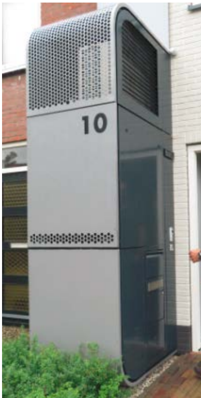
Figure A30. Exterior mechanical shed in the front yard
