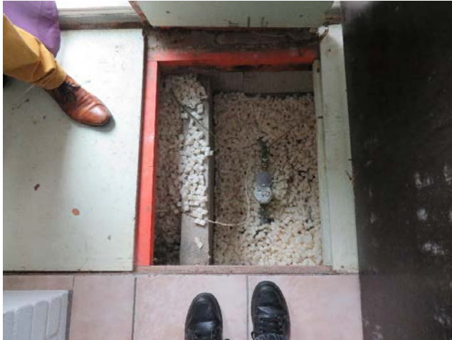
Figure 20. Crawlspace insulated with polystyrene chips
