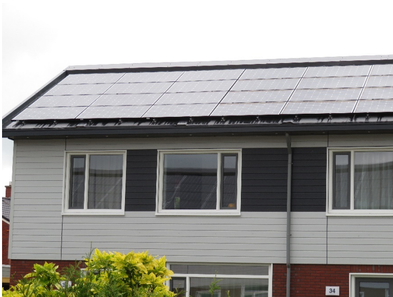
Figure A18. Solar modules
