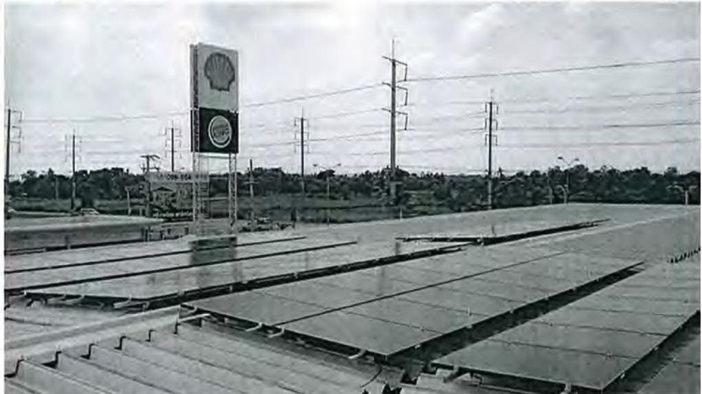
Solar panels are installed on the rooftop of a Shell service station in Thailand.
