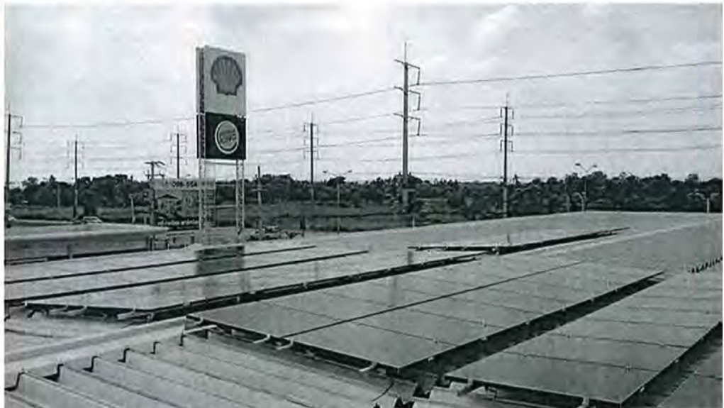
Solar panels are installed on the rooftop of a Shell service station in Thailand.
