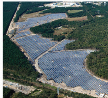
Long Island Solar Farm Brookhaven National Laboratory
