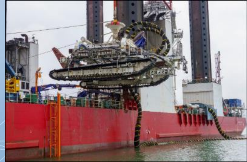
Tracked Trencher Van Oord's 'Deep Dig-It' Weighs 125T, jetting and chain cutting up to 5.0m burial depth
