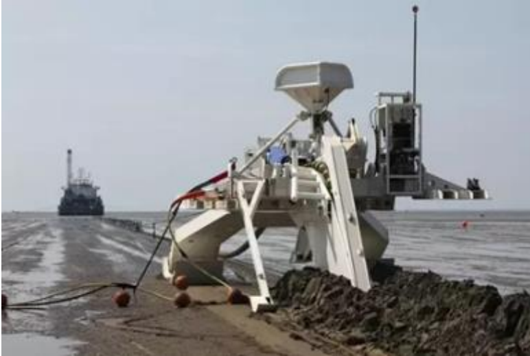
Towed Plow ~3m/10' burial depth 15m long, 6.5m wide Weighs approx. 50T
