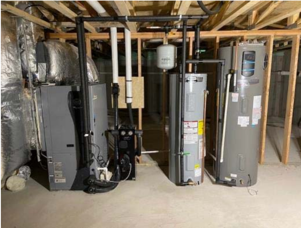
Photo of the Project GSHP setup at the Medford Site with equipment from left to right consisting of the WaterFurnace® 7 Series, flow center, domestic hot water tank, and landlord-provided hybrid electric water heater.
