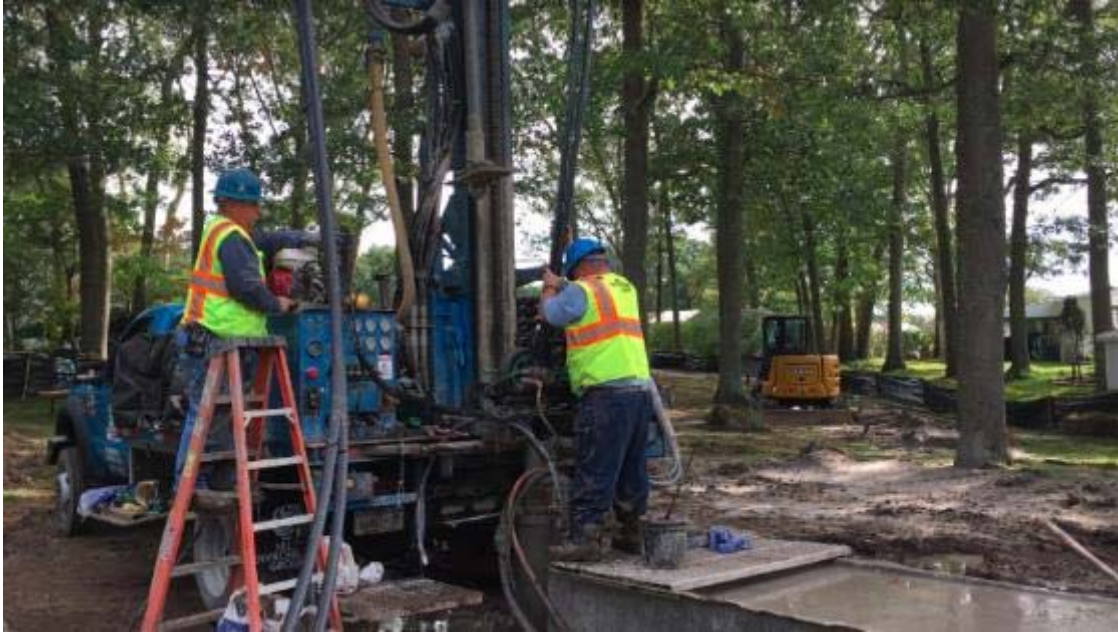
Photo of the geothermal pipes being installed after well boring completion at the Glenwood Village Site.
