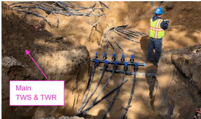
Figure 18. Photos Showing Header Details from Ground Loop Heat Exchanger to Each HP
