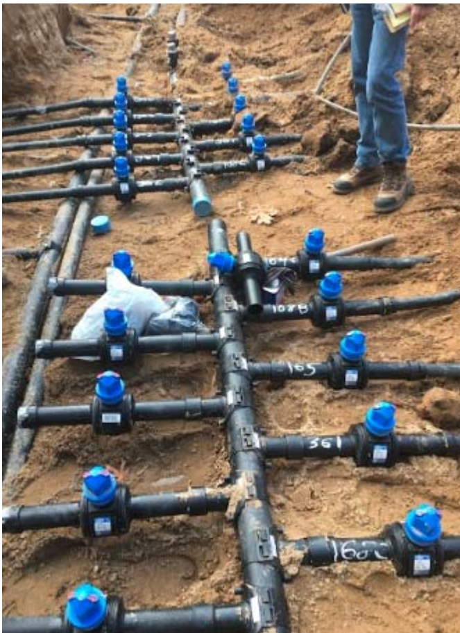
Photo of the pipe headers and valves in the community part at the Glenwood Village Site.
