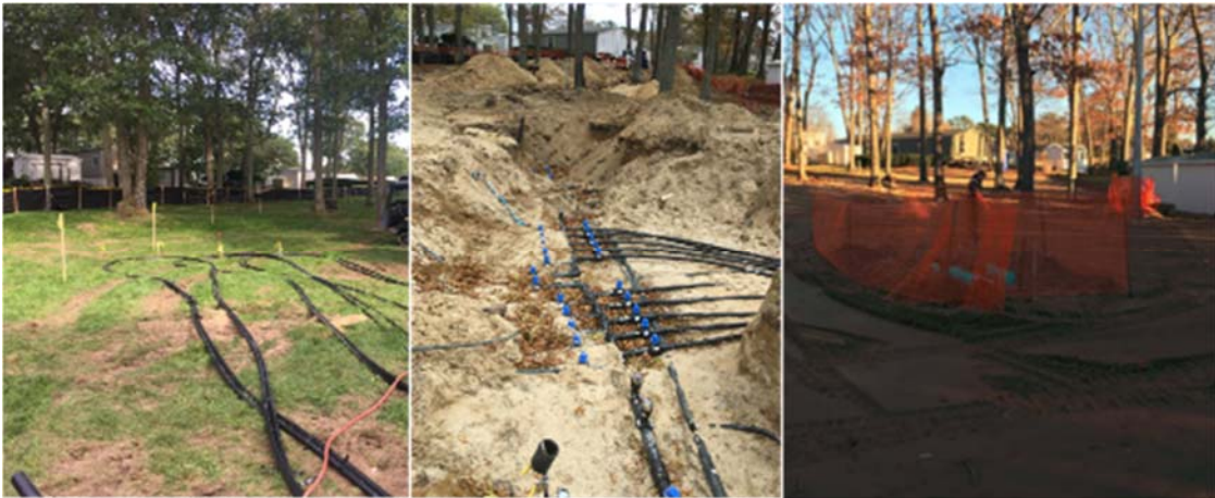
The community park at the beginning of construction, midway after pressure testing, and final landscape restoration at the Glenwood Village Site.
