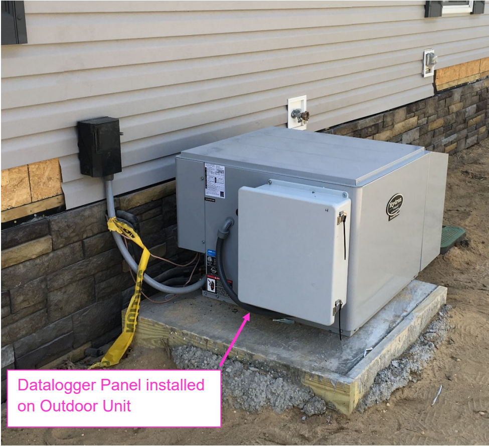
Figure 2. Outdoor Section of “Split” GSHP Unit (RT series)
