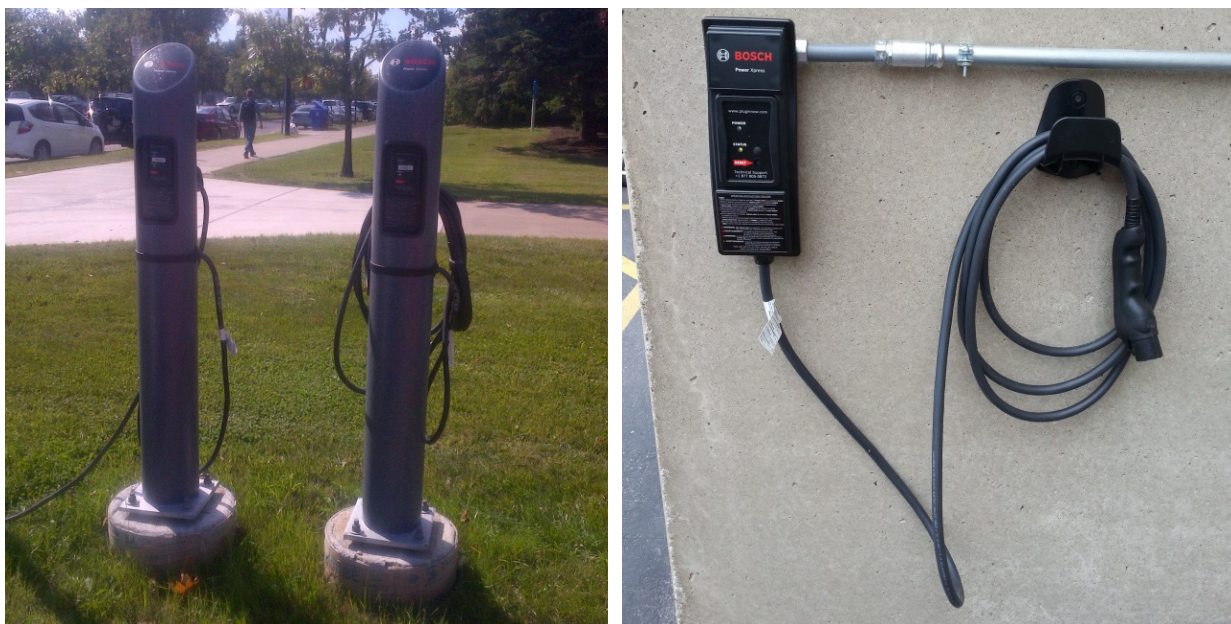
Figure 4. Non-networked Level 2 Charging Stations Installed for BCS EVs
