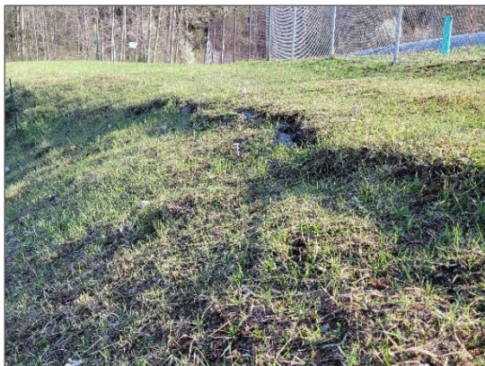
Figure 4-1. North Slope – April 2021 Pre-Movement.
