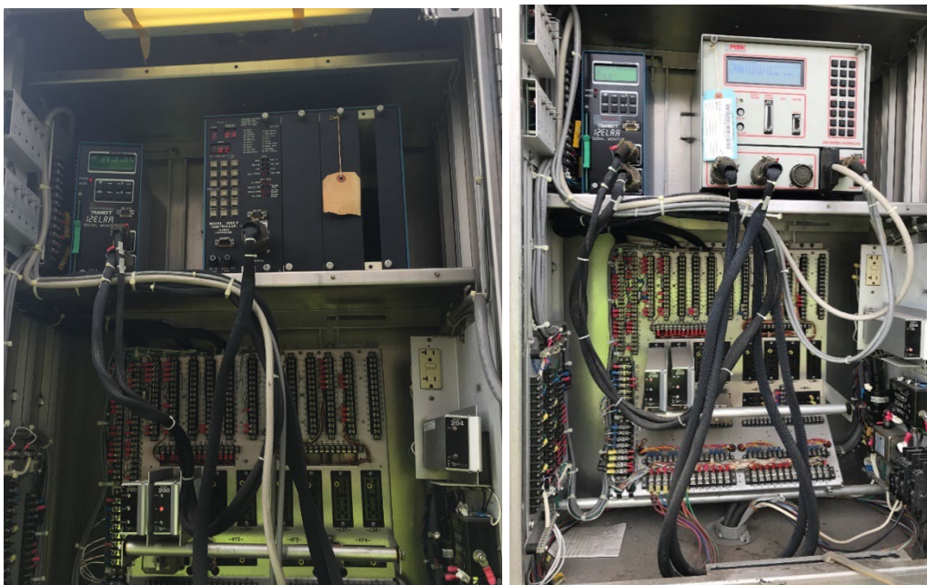
Figure 4. Cabinet Equipment for Sydney Avenue (left) and Oakley Avenue (right)
