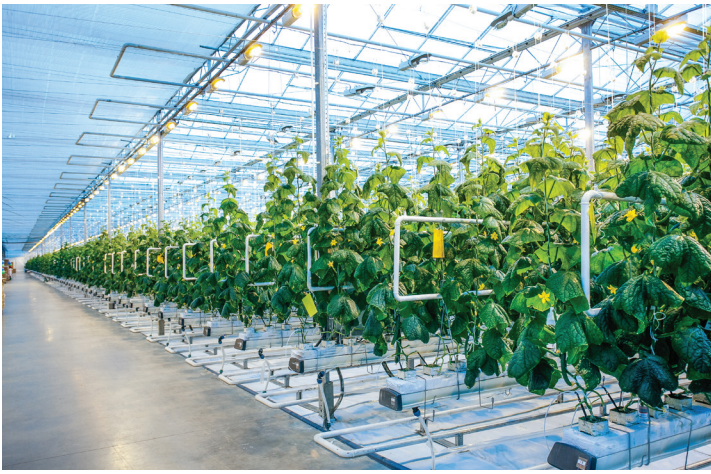
Crop Bottom Heating with Hot Water Systems
