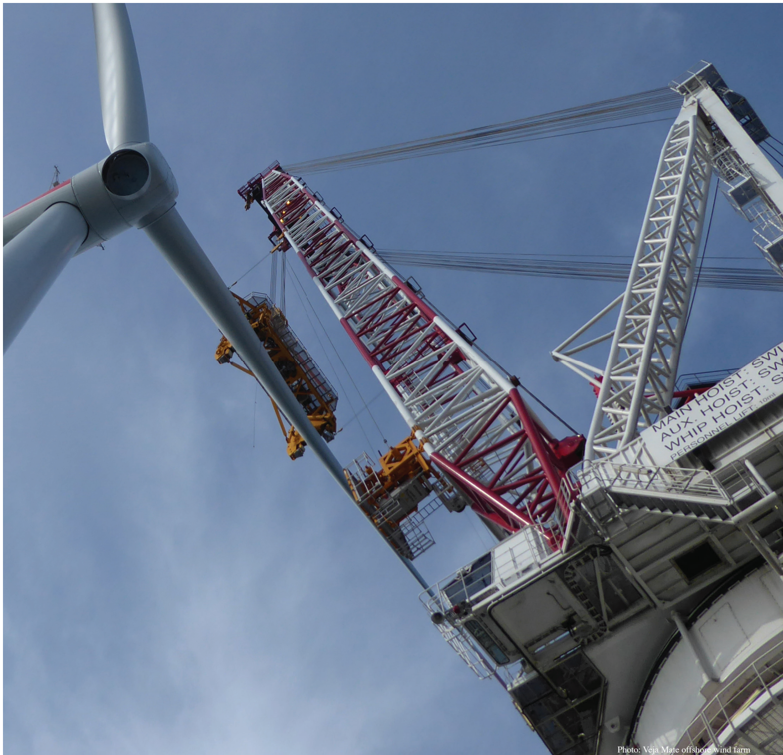
Photo: Veja Mate offshore wind farm
