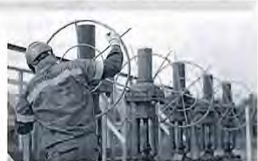
An employee working at the Solyim Petroleum JV in Russia.
