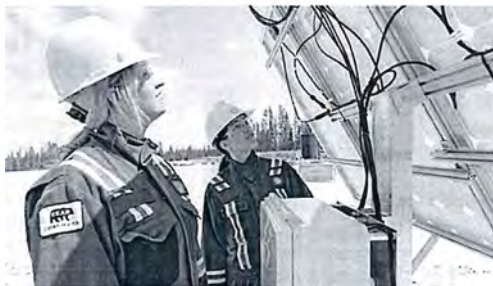
We have installed methane detection technology at our unconventional gas project near Rocky Mountain House, Canada.
